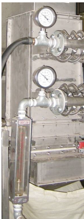
Fig. 4 – Water Manifolds and Instrumentation
